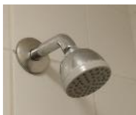
Figure 9. Low flow shower heads installed
